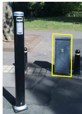
External feeder pillar
