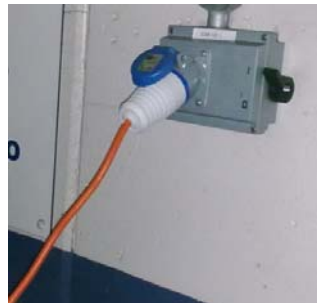
Blue commando connected to an open access charging point
