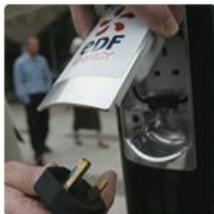
3-pin plug socket on restricted access charging point
