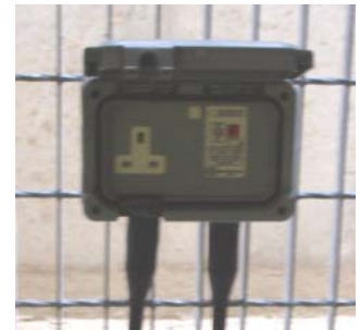
3-pin plug socket on open access charging point
