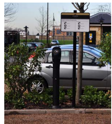
Off-street restricted access charging point in car park
