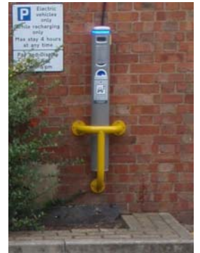
Wall mounted charging point with protective cage
