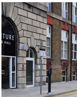
Cadogan Road, Woolwich Integrated feeder pillar within the EVCP post (Source: Infracharge Ltd)
