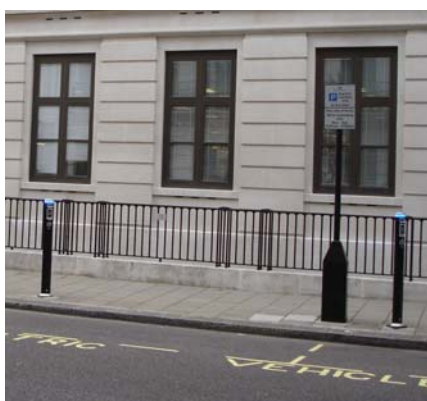
Wilton Street, Westminster Integrated feeder pillar with signpost
