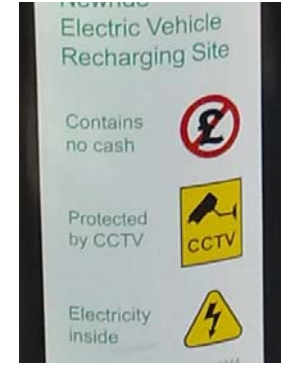
LB Islington – charging point contains warning notices (eg 'protected by CCTV')
